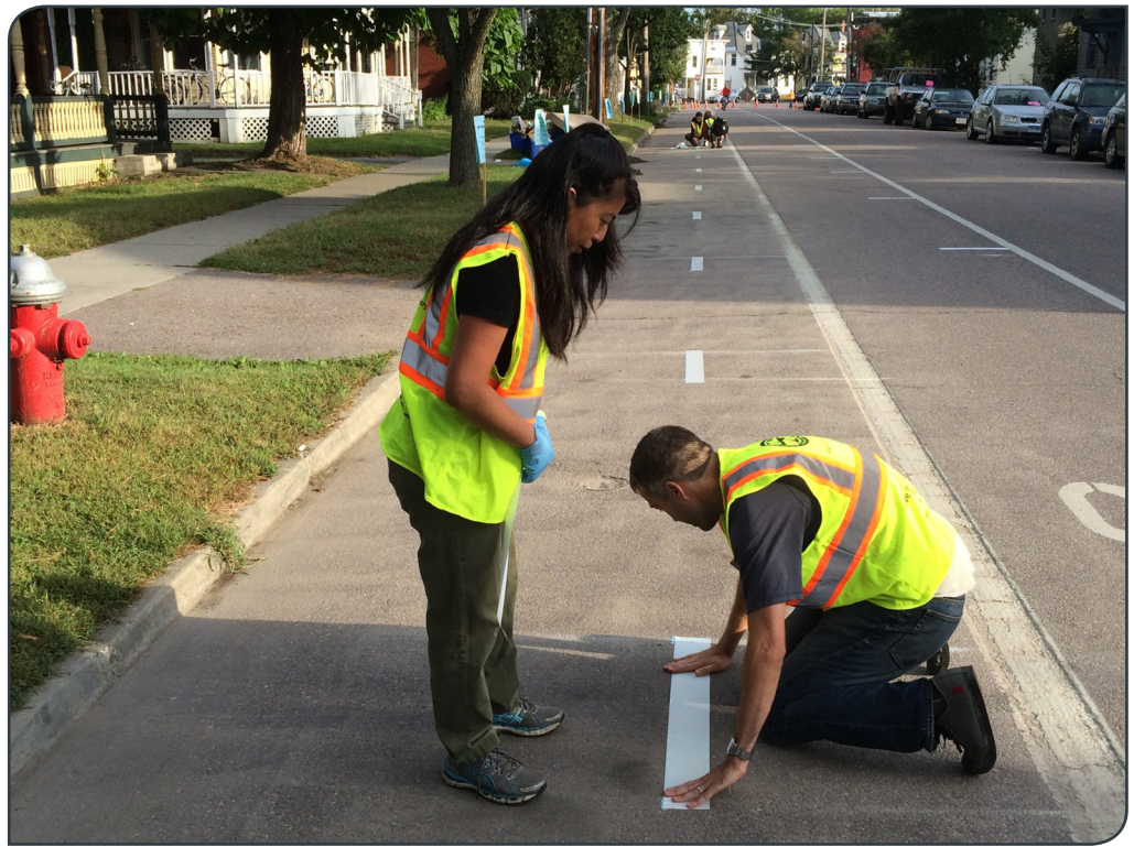
Using duct tape, these volunteers are creating a pop-up buffered bike lane in Burlington, Vermont. Photo: Street Plans Collaborative
