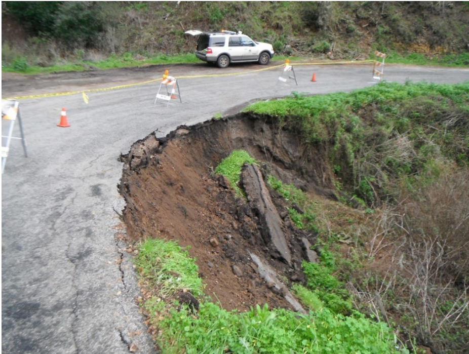
Slope failure with pieces of pavement falling down slope
