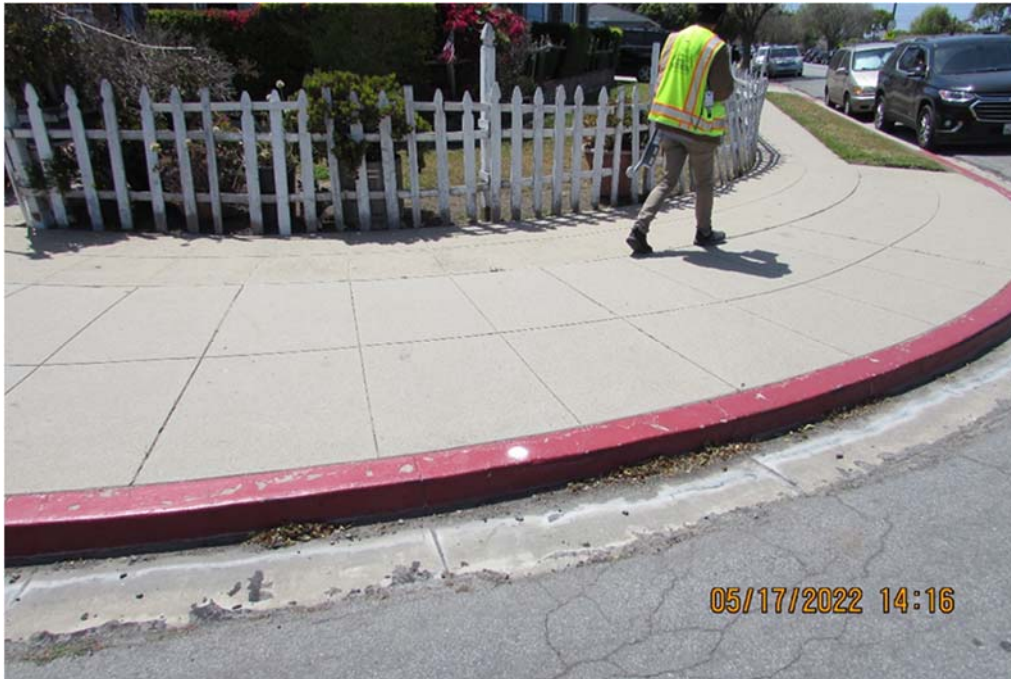
Before photo of W Acacia St Citywide Sidewalk Repair Project
