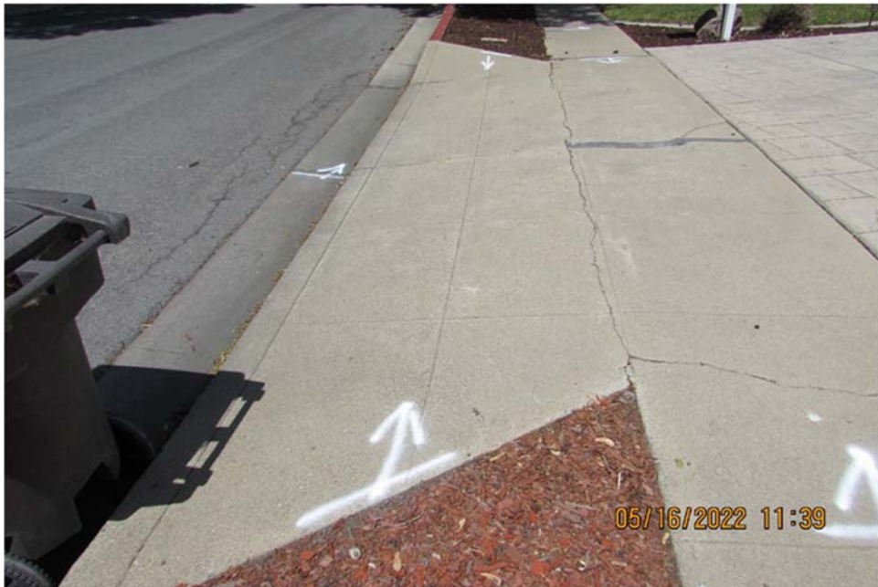
Before photo of San Miguel Ave Citywide Sidewalk Repair Project
