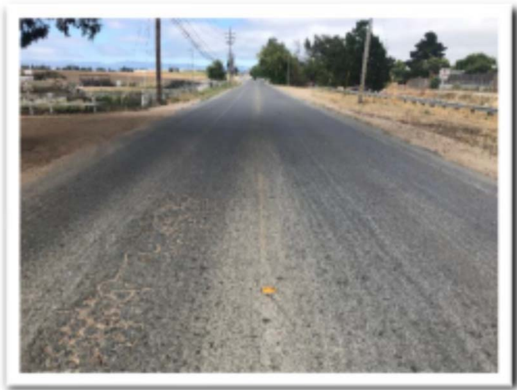
Before: San Juan Grade Road @ ~1,500' North of Van Buren Avenue facing South
