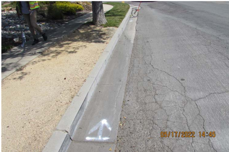
Before photo of San Vicente Ave Citywide Sidewalk Repair Project
