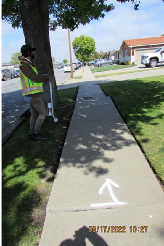
Before photo of W Acacia St Citywide Sidewalk Repair Project
