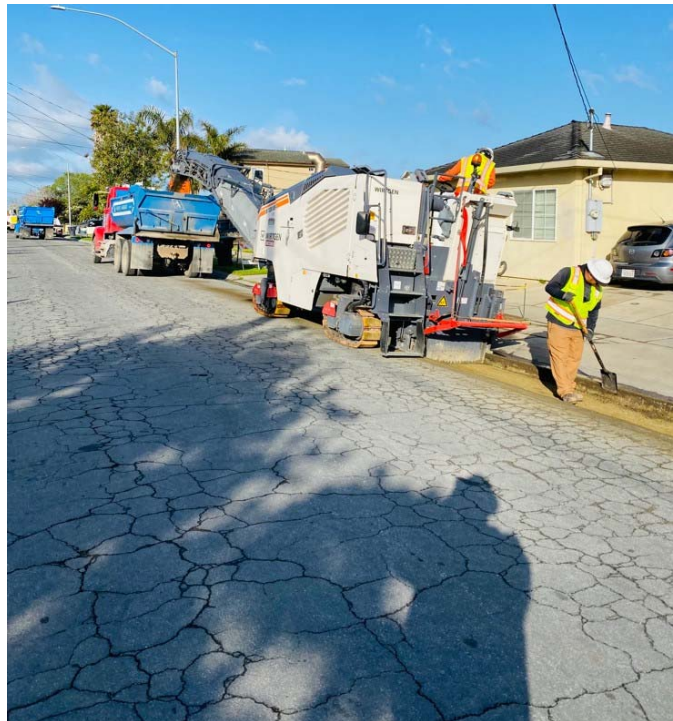
Dallas Ave between Del Monte Ave and Cortez St during beginning of construction.
