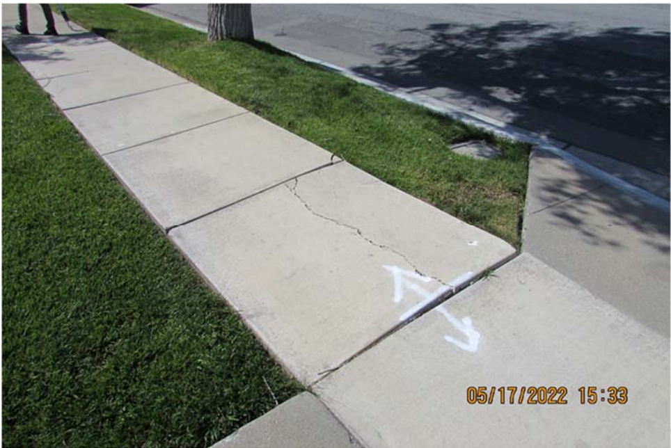
Before photo of Palma Dr Citywide Sidewalk Repair Project
