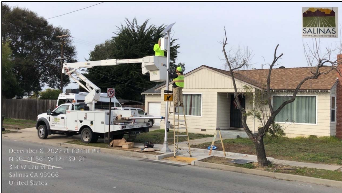
Construction Photo: Installing the Pedestrian Hybrid Beacon at W Laurel Drive at Parkside Street
