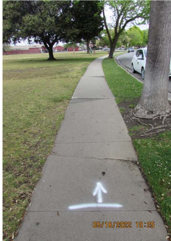
Before photo of San Miguel Ave Citywide Sidewalk Repair Project
