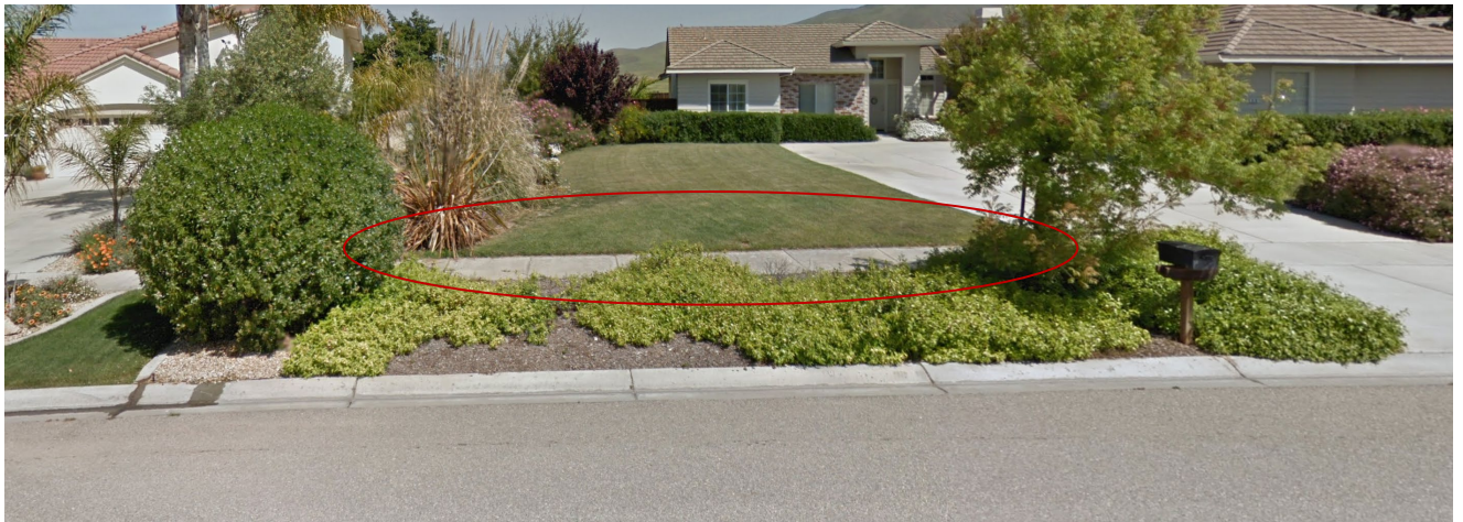
Before Picture: 359 Blueridge Ct – Property Owner Had Severe Cases of Spalling Along the Sidewalk Panels Located Adjacent to the Property.
