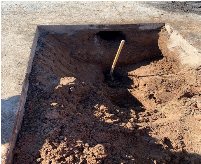
Before Picture: Monterey Street - Initial Cut and Attempt of Repair Before Staff Discovered the Tunnel-Like Path Found Under the Existing Pavement.
