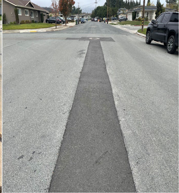
After Picture: Soledad Street – Post Pavement Repair of the Destablized Road Segement
