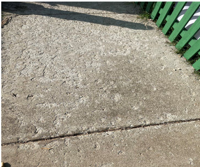
Before Picture: 359 Blueridge Ct – Spalling Close Up
