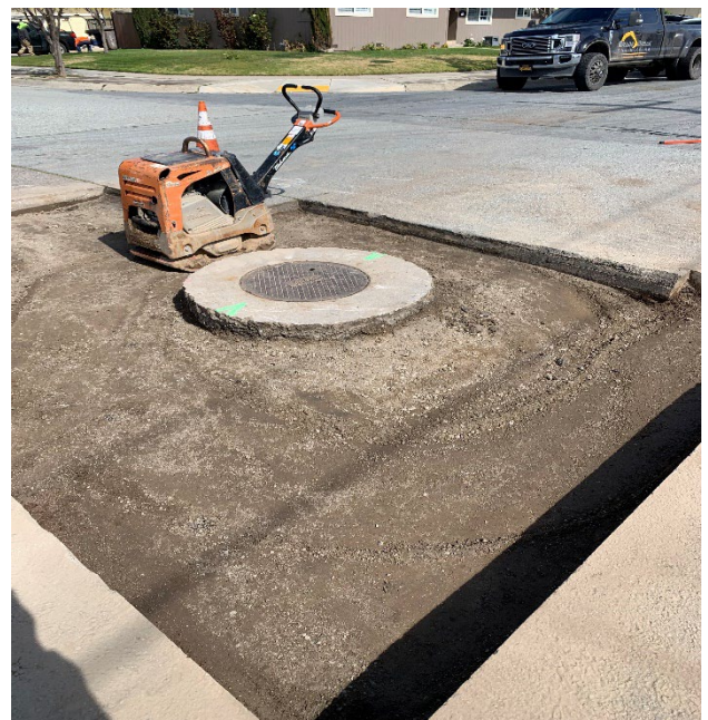
Before Picture: Soledad Street – Area Around the Manhole That Required Repair.
