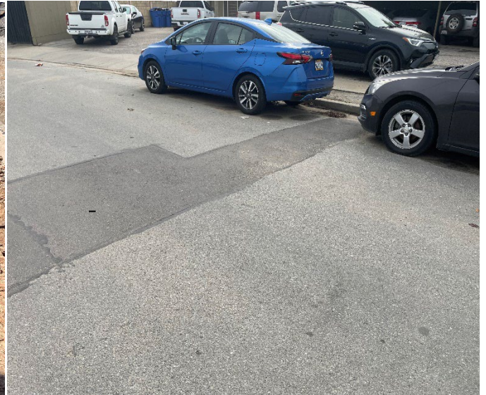
After Picture: Monterey Street - Post Pavement Repair of the Water Damage on Monterey Street.
