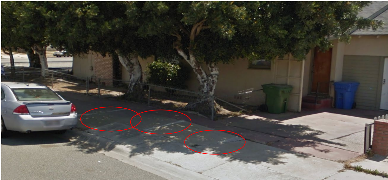
Before: 1200 Palm Ave – Property Owner Replaced Concrete Sidewalk Panels That Were Raised due to Tree Roots
