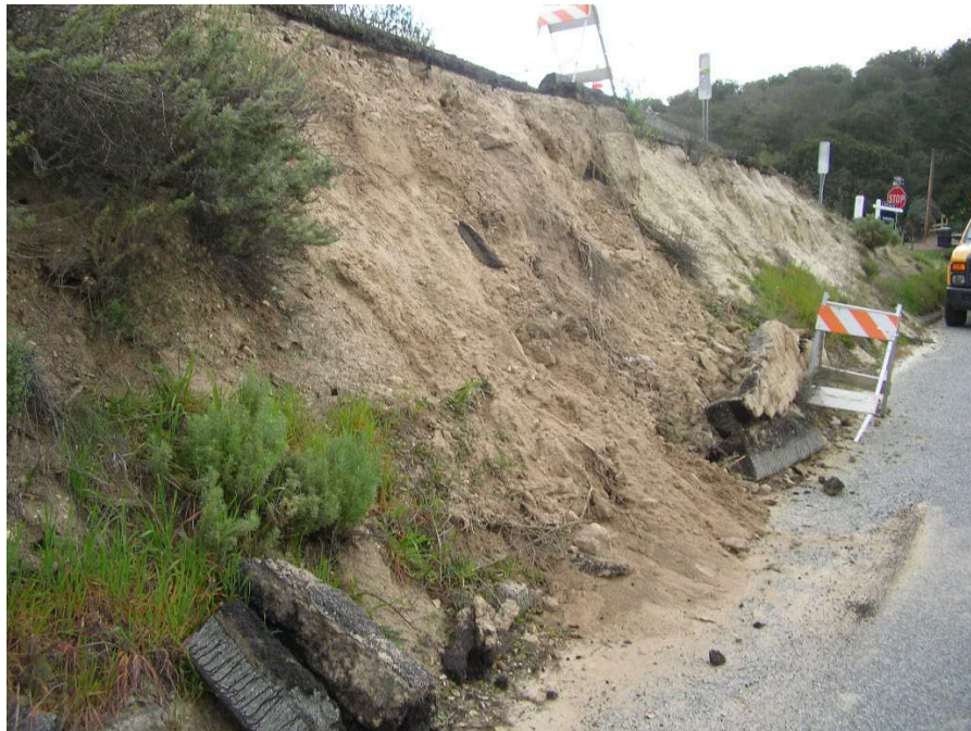
Slope failure with pieces of pavement falling onto adjacent road
