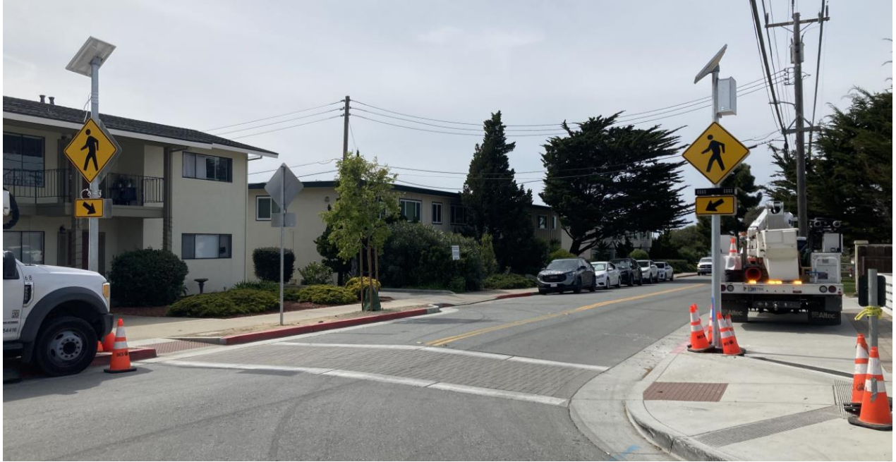
After Rectangular Rapid Flashing Beacon Installed, 2023
