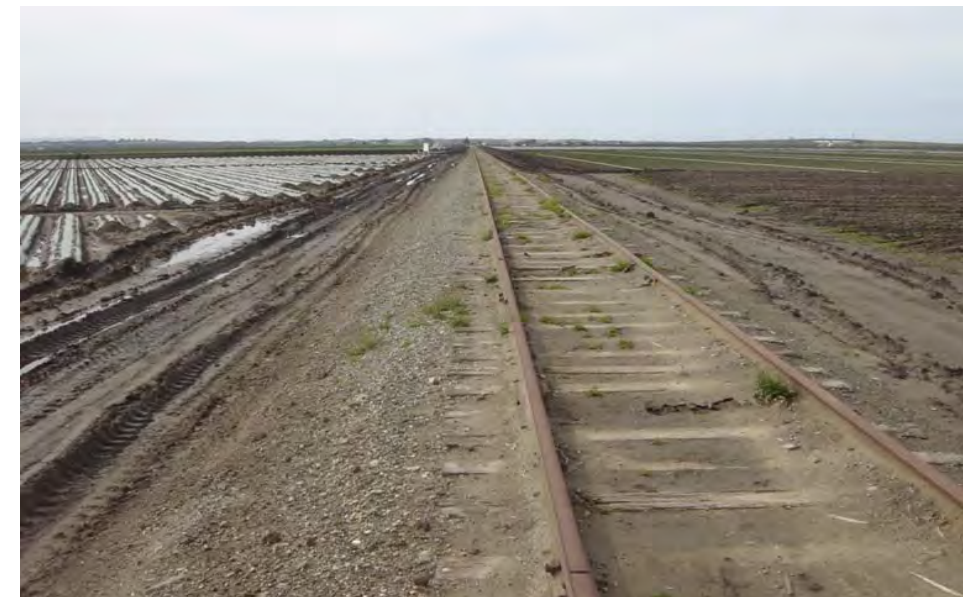
Figure 9-36 Ponding along the Edge of Rail Looking South
