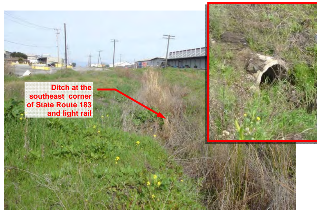
Figure 9-27 Ditch at the Southeast Corner of State Route 183 and Light Rail Looking North
