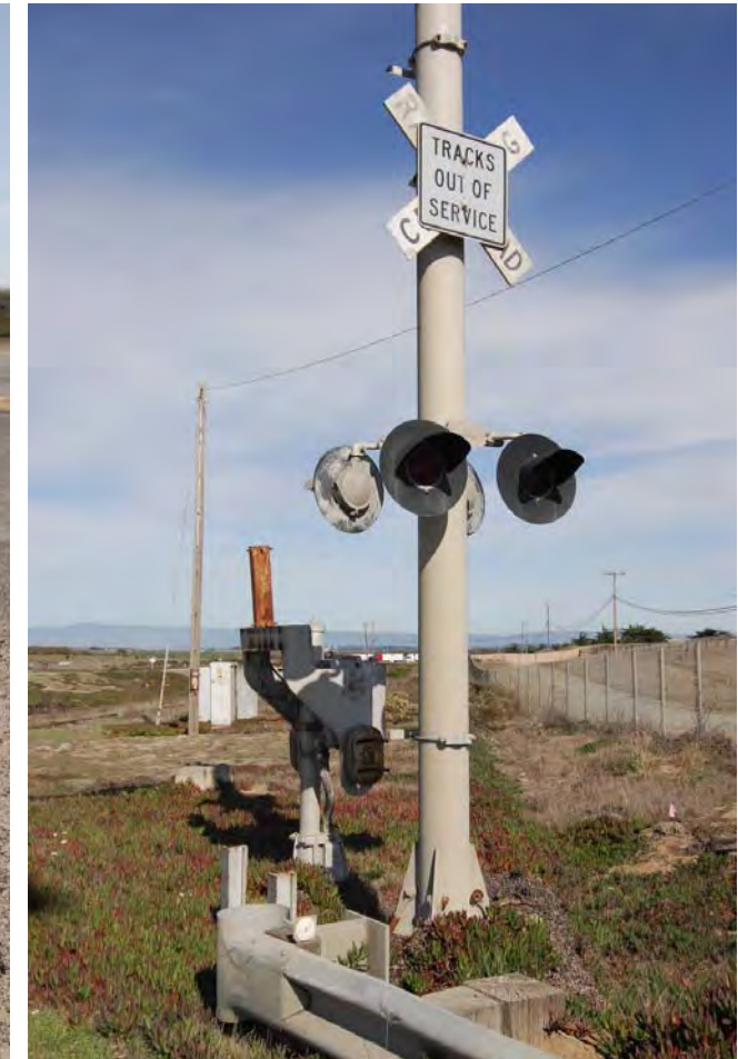
Non-Functional Controls at Del Monte Boulevard (MP 114.30)
