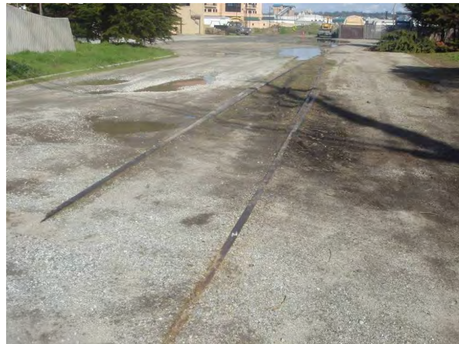
Figure 9-81 Ponding North of Contra Costa Street Crossing
