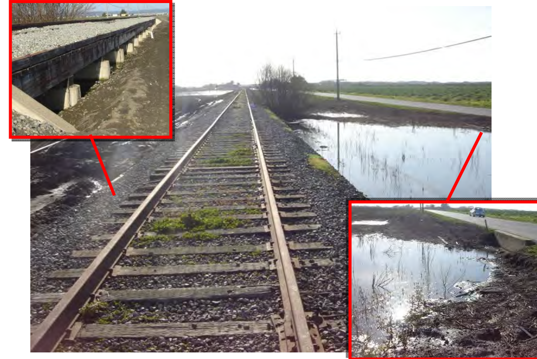
Figure 9-48 Ponding at Equalizer Trestle Bridge at MP 112.8
