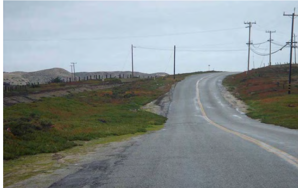
Figure 9-62 Low Elevation Area on Lapis Road around Station 256+00
