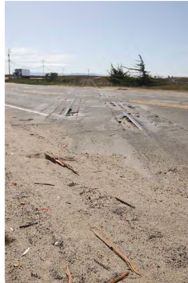
Track Condition at Del Monte Boulevard (MP 114.30)
