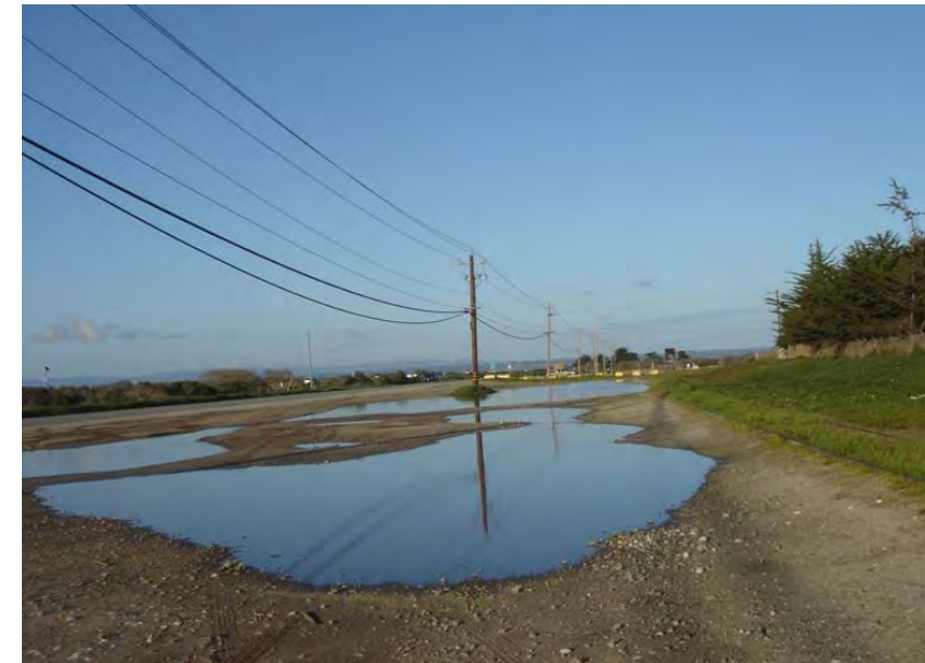
Figure 9-56 Ponding between South Dole and North Dole Entrances
